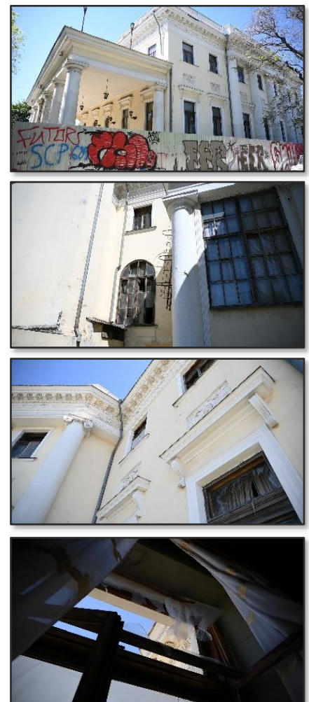
Figure 68. Visible lateral damage presence on the Vorontsov Palace (Credit: Odesa City Council, 2022)
